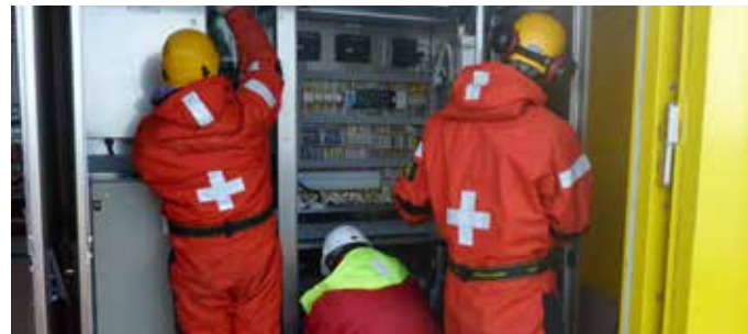
Replacing and Calibrating Equipment
